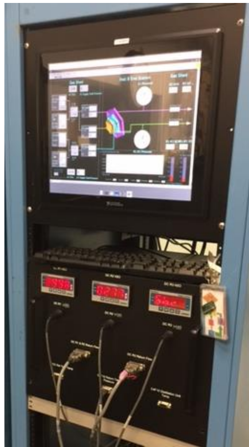
Custom controls interface chassis with touchscreen monitor
